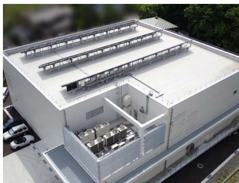
Solar panels installed on the roof of the warehouse building at the Wakaho Plant
