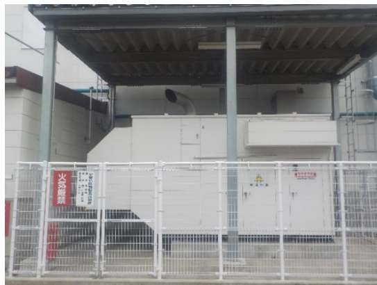
Emergency power generator (Arai Plant)
