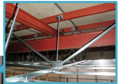
Aseismic frame in the ceiling
