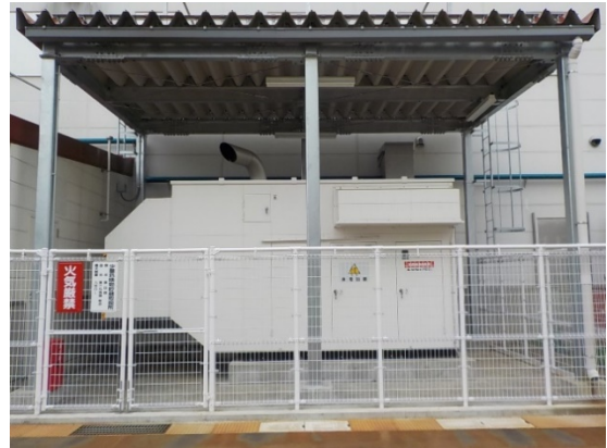
Emergency power generator
