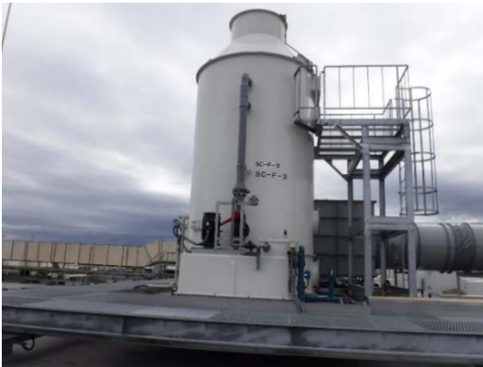
Exhaust gas scrubber
