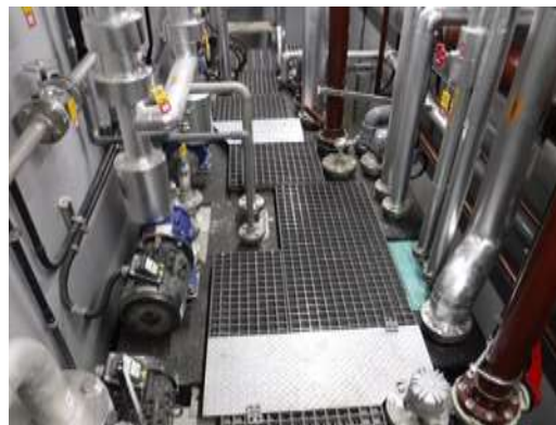
Plating pre-treatment equipment
