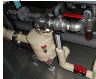
Waste heat recovery heat exchanger
