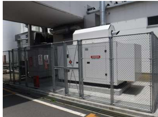
Emergency power generator
