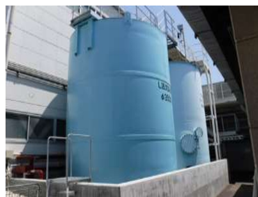
Updated wastewater treatment equipment
