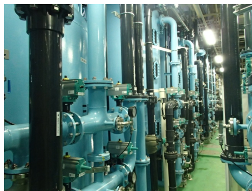
Upgraded recycling water equipment at the Takaoka Plant
