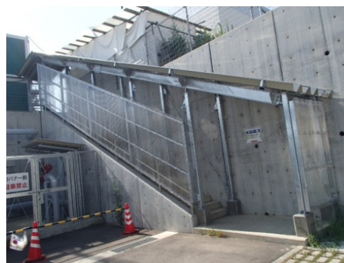
The roof and snow fence that were installed on the inspection route
